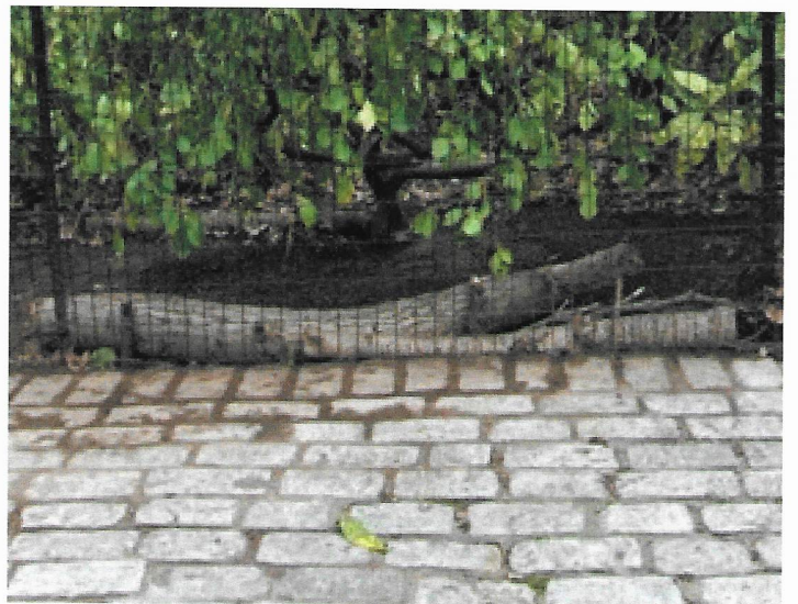
Top: Erosion mitigation in-progress; Middle: New coir logs Bottom: An example of cribbing logs
